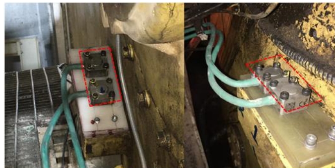
Figure 4. Placement of CA 202 accelerometer sensors throughout various sections of the gas turbine at the Kirkuk power plant.
